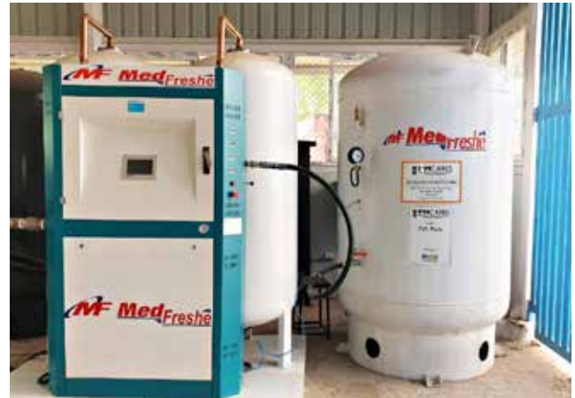
PSA plant of 1000 LPM installed at ESIC Model Hospital, Ludhiana
